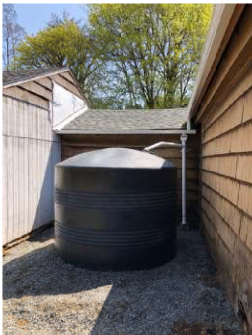
New rainwater catchment tank at Marys River Grange.
